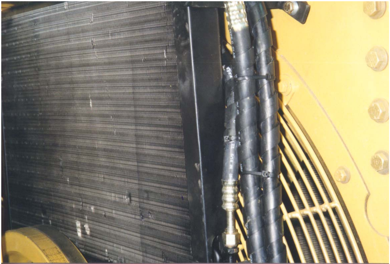
Right side of condenser with hoses in place.
