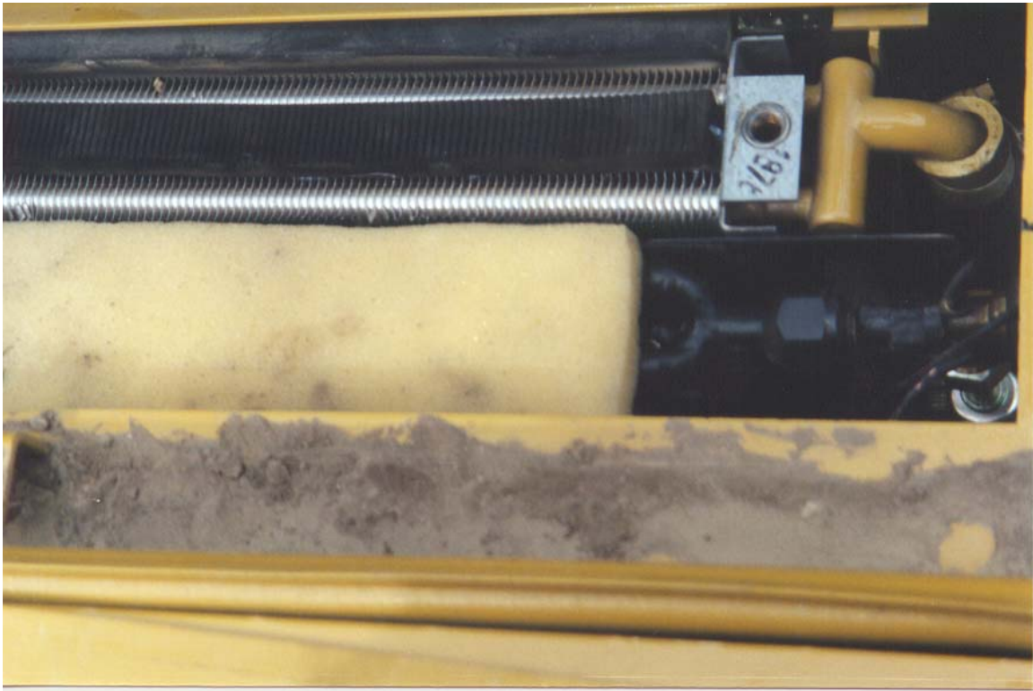
Top of evaporator assembly in heater box.
