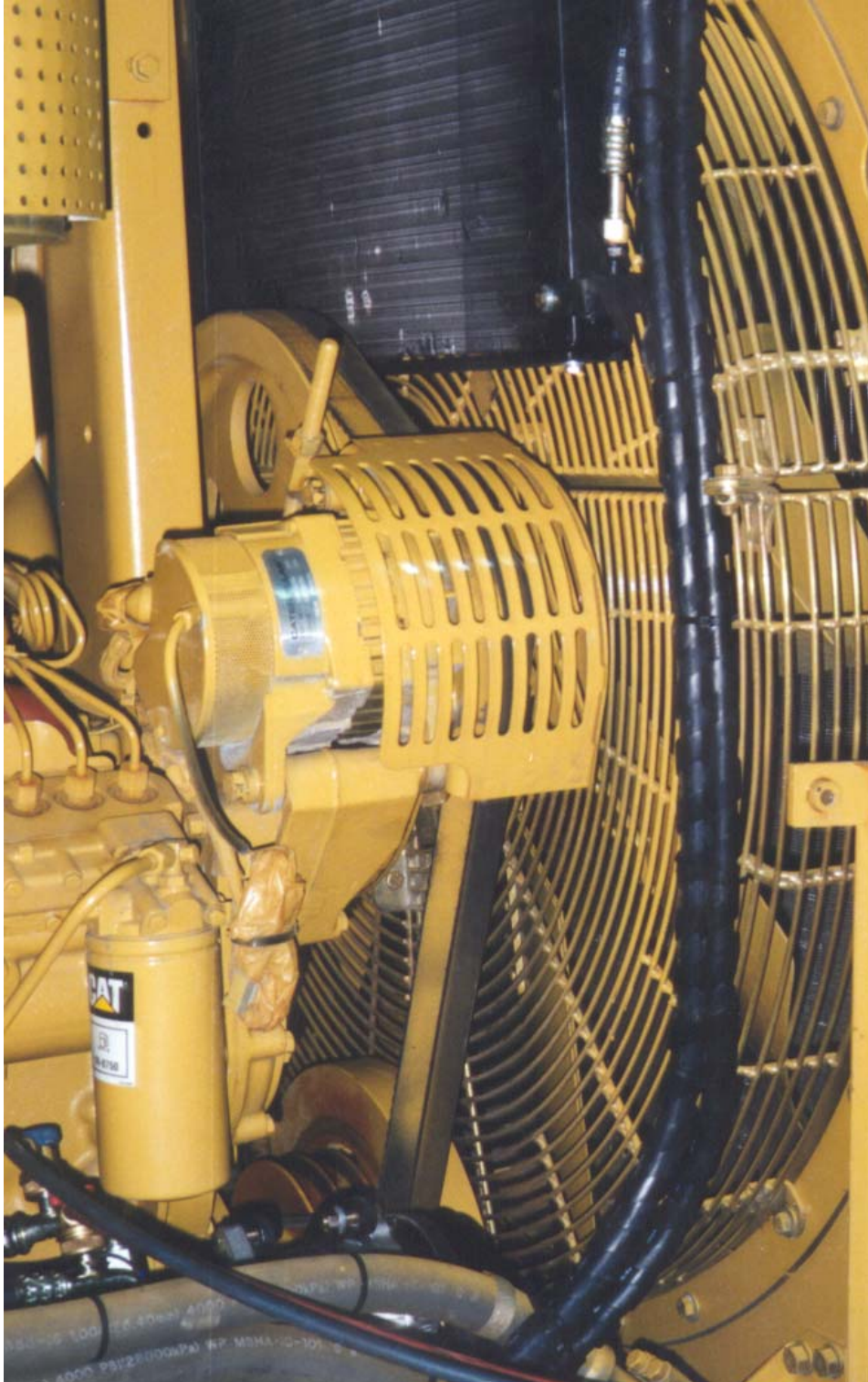
Hose routing at condenser down radiator screen.
